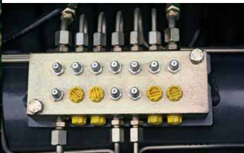
All lubrication points are grouped on a bank.
