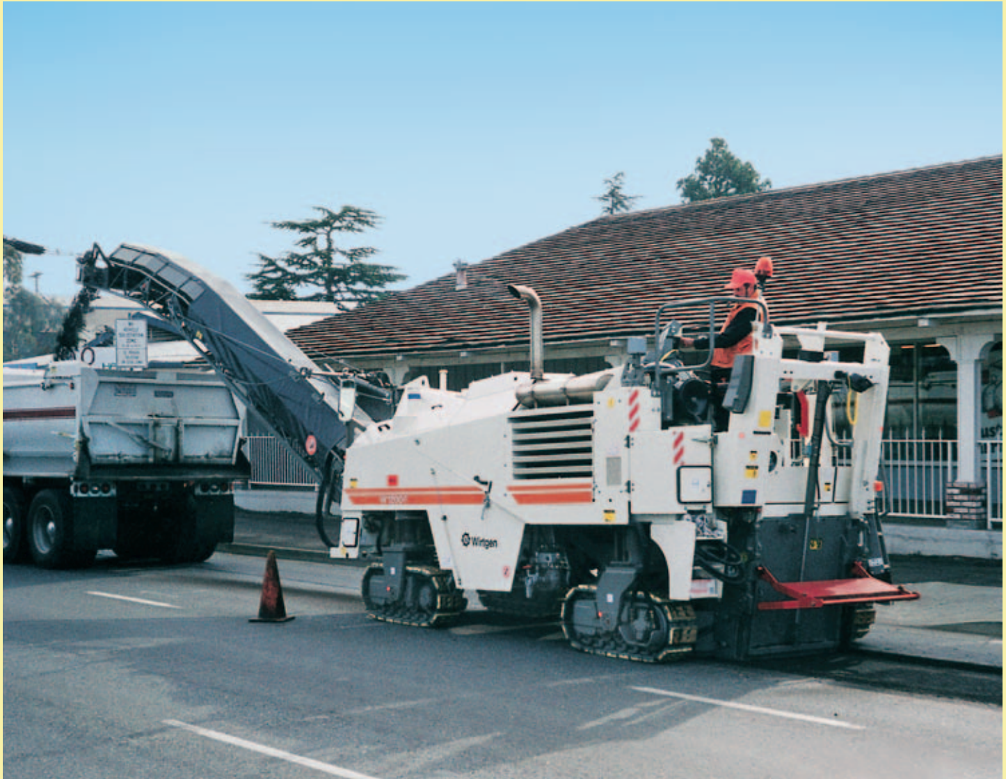
W 1200 F milling off the surface course of an urban road in the USA. The machine leaves a neat milled surface, despite its considerable rate of advance.
