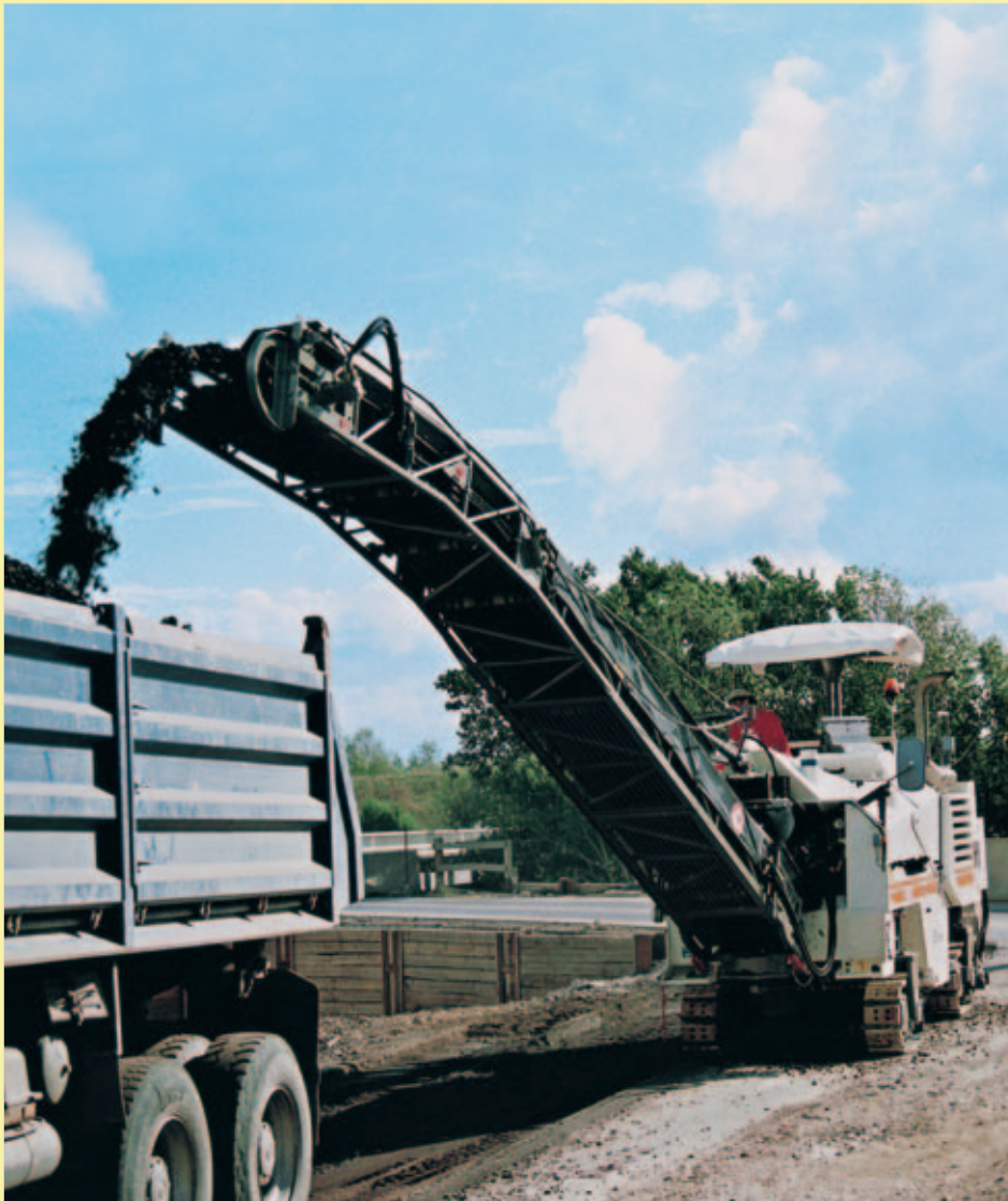
The slewing discharge belt allows the milling machine operator and truck driver to adjust precisely to the conditions prevailing on site.
