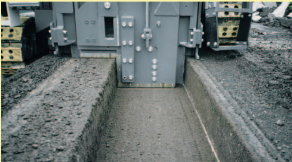
Milling unit of a W 1200 F with 60 cm wide milling drum digging a trench for cables. The left-hand crawler is travelling on ground of limited bearing capacity.
