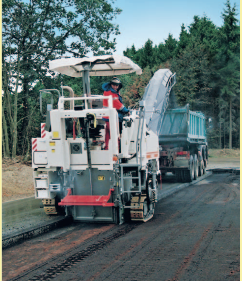
The entire pavement is removed by the W 1000 F, track for track. The crawlers ensure good traction and safe operation on the loose substrate, as well as a rapid rate of advance.
