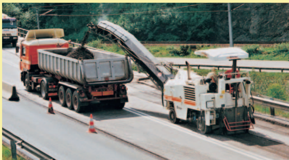
The wheel-mounted W 1000 F or W 1200 F is ideal for removing individual asphalt courses, for instance when rehabilitating stretches of road within towns and cities.
